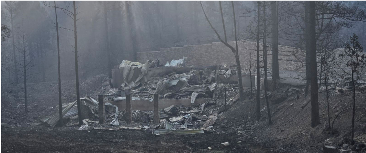
Figure 9: Image of Post-Fire Home Damage (Lincoln County)
