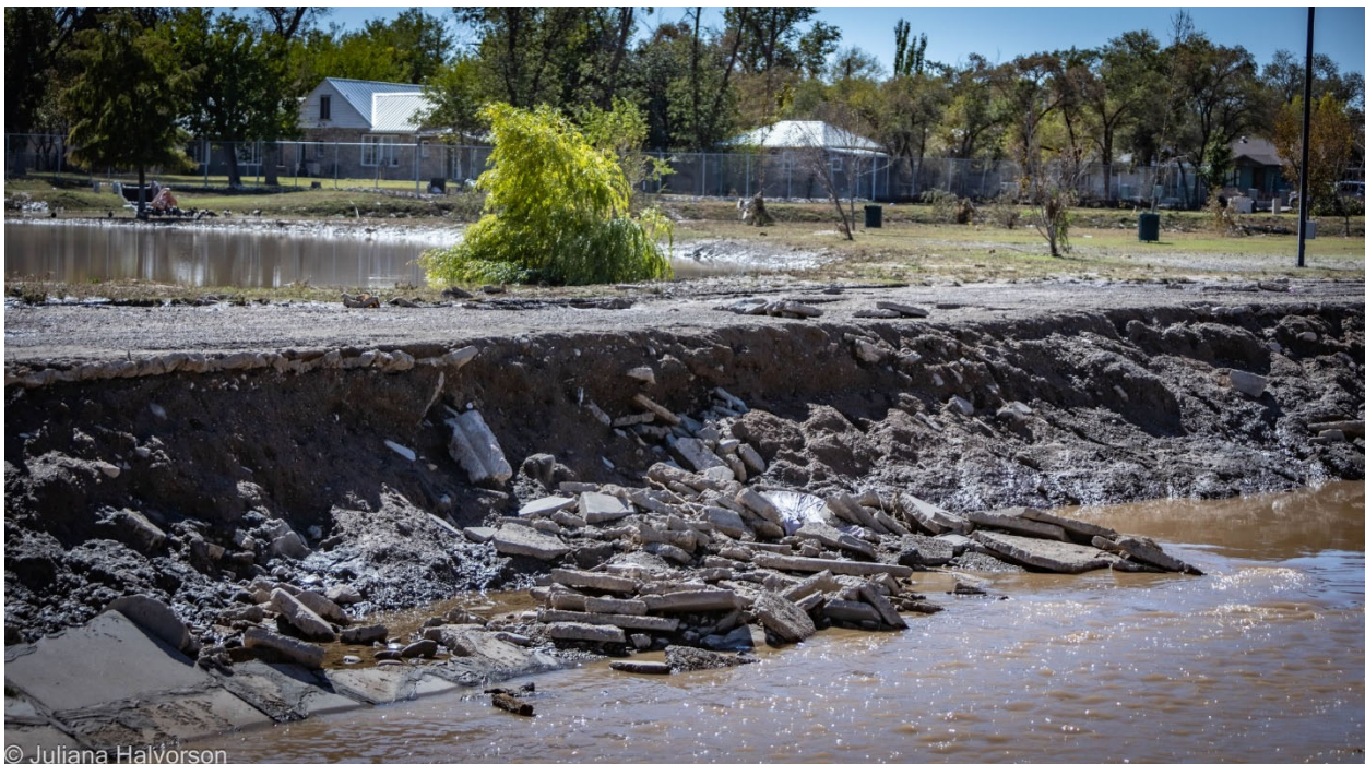
Figure 11: Image of Waterway Damage (Chaves County) Photo Credit: Juliana Halverson
